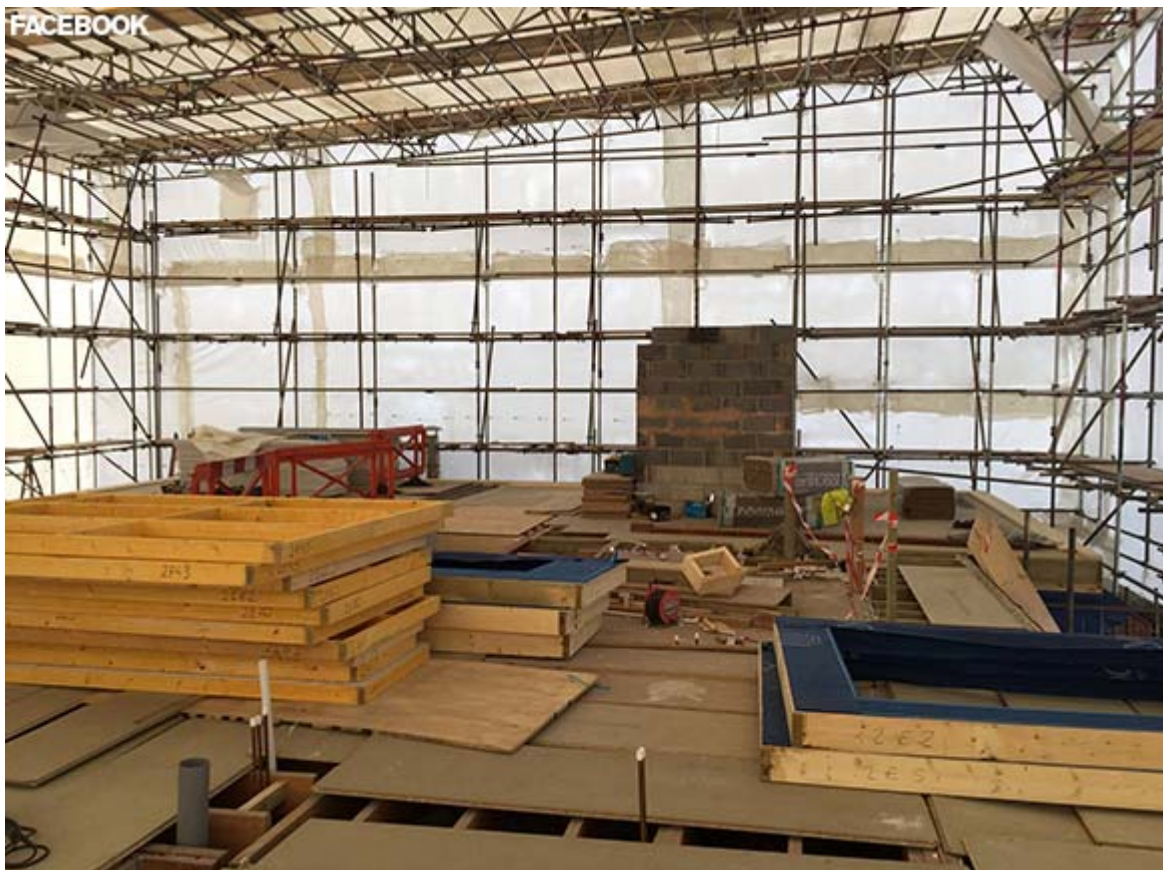
The company was served an improvement notice after workers in a loft
