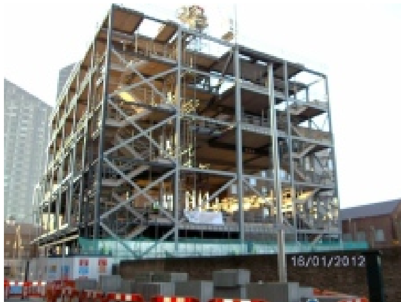
Fifteen days before collapse
