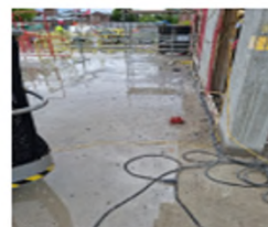
Concrete debris fallen from slipform.
