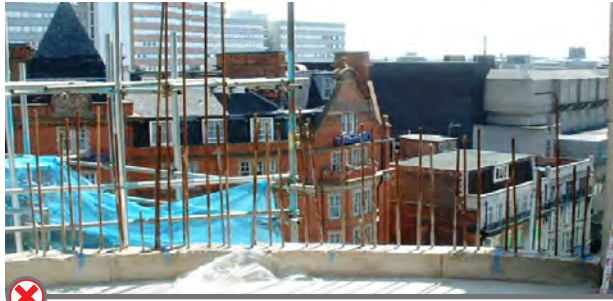
Only the rebar is preventing a fall.
